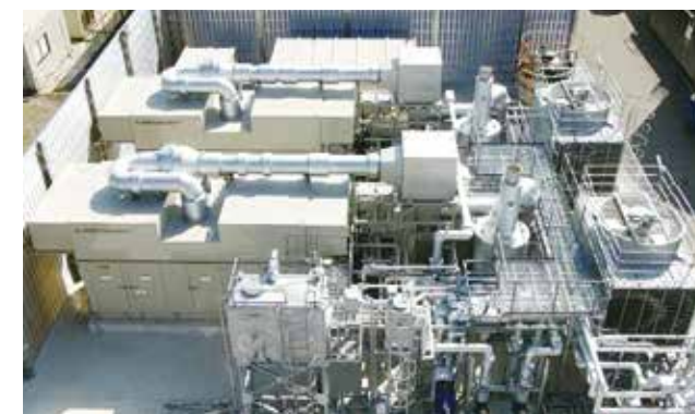
Cogeneration facility with a total output of 2,000 kW
